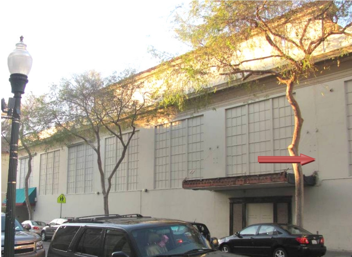
South elevation, view looking northwest across Kittredge. Note full height crack in wall where 1913 and 1926 additions meet. (Architectural Resources Group, December 2013)
