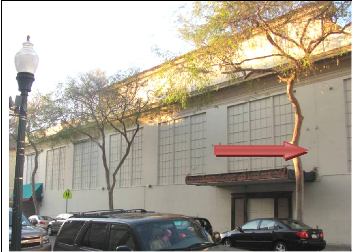
South elevation, view looking northwest across Kittredge. Note full height crack in wall where 1913 and 1926 additions meet. (Architectural Resources Group, December 2013)
