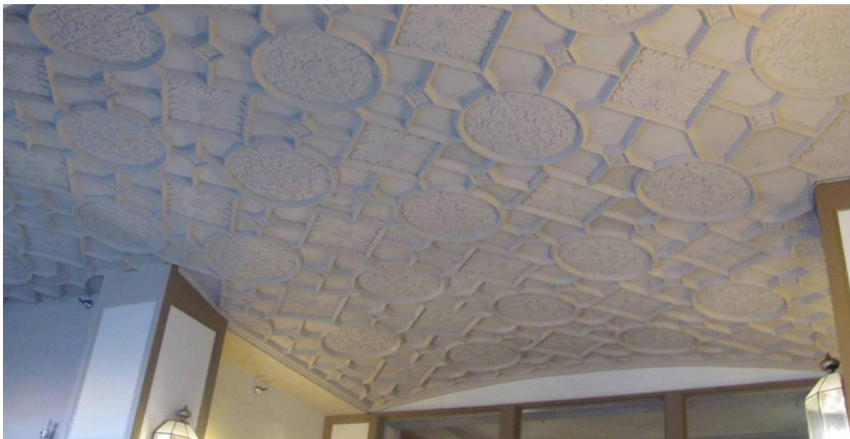
Portion of decorative plaster ceiling remaining from original Hink's Department Store entry arcade (now entrance to cinema) (Architectural Resources Group, December 2013)
